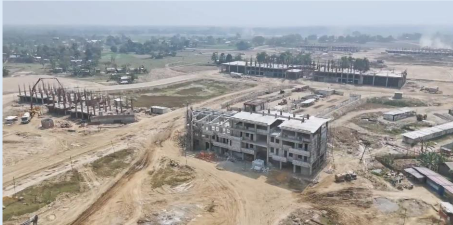
The status of the main campus situated at Mangaldai as on 20 th March 2024. The campus is expected to be ready by August 2025
